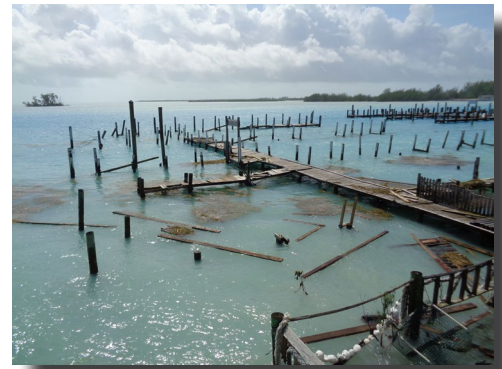
Marina damage in Alice Town
